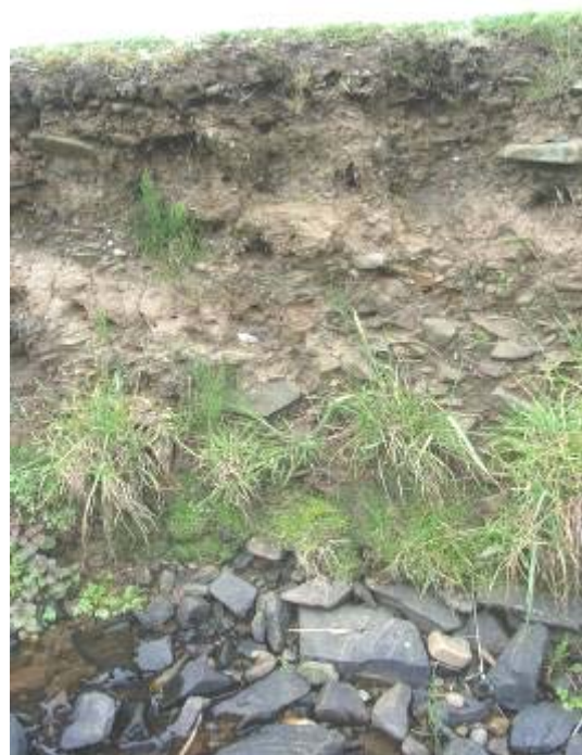
Figure 17: Erosion of bank on the valley stream looking south
